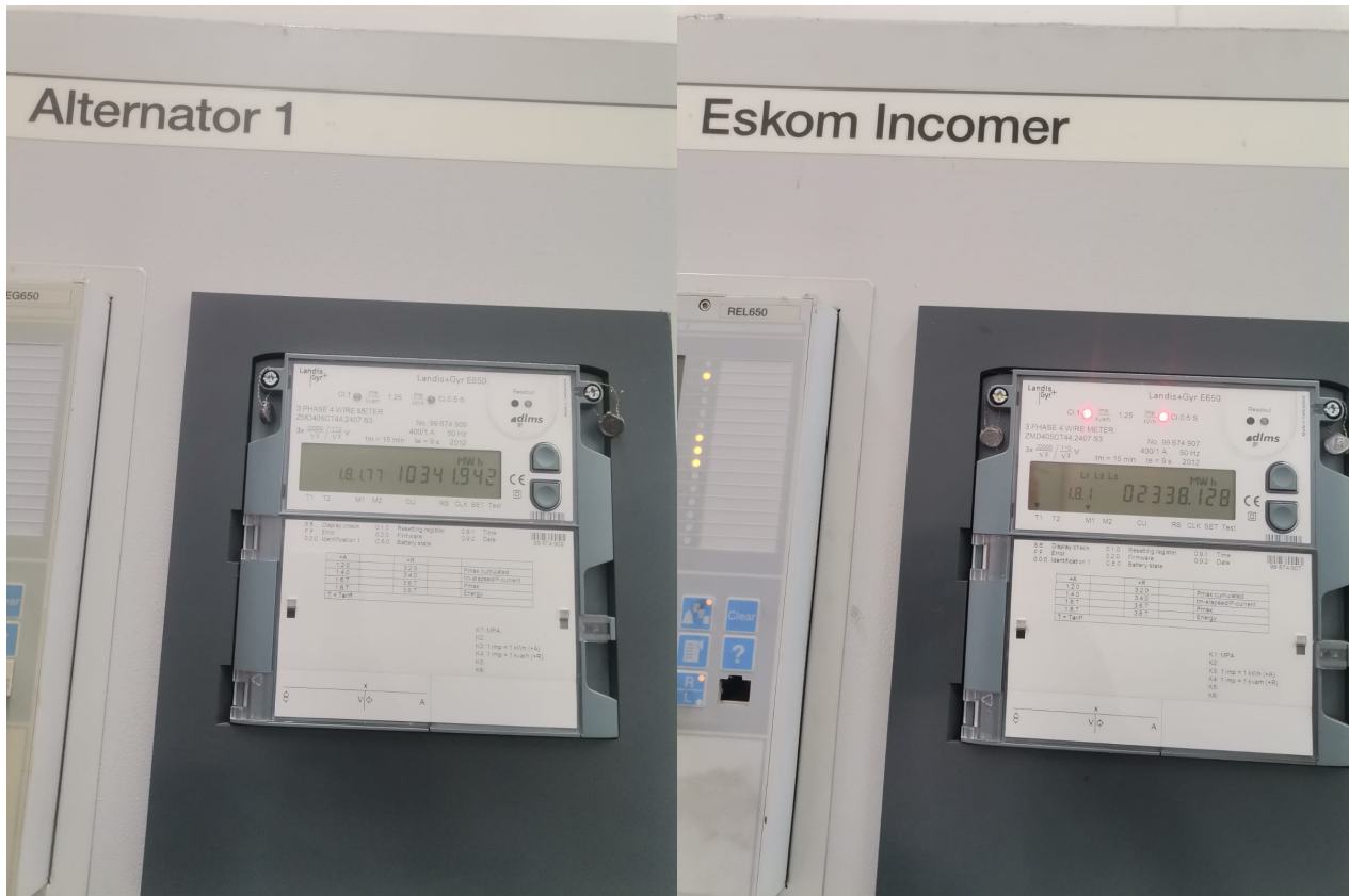
Figure 1 Example of metering device for TA 1 and Eskom incomer.
